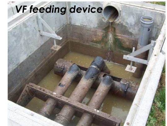
Special siphon for energy-free feeding
